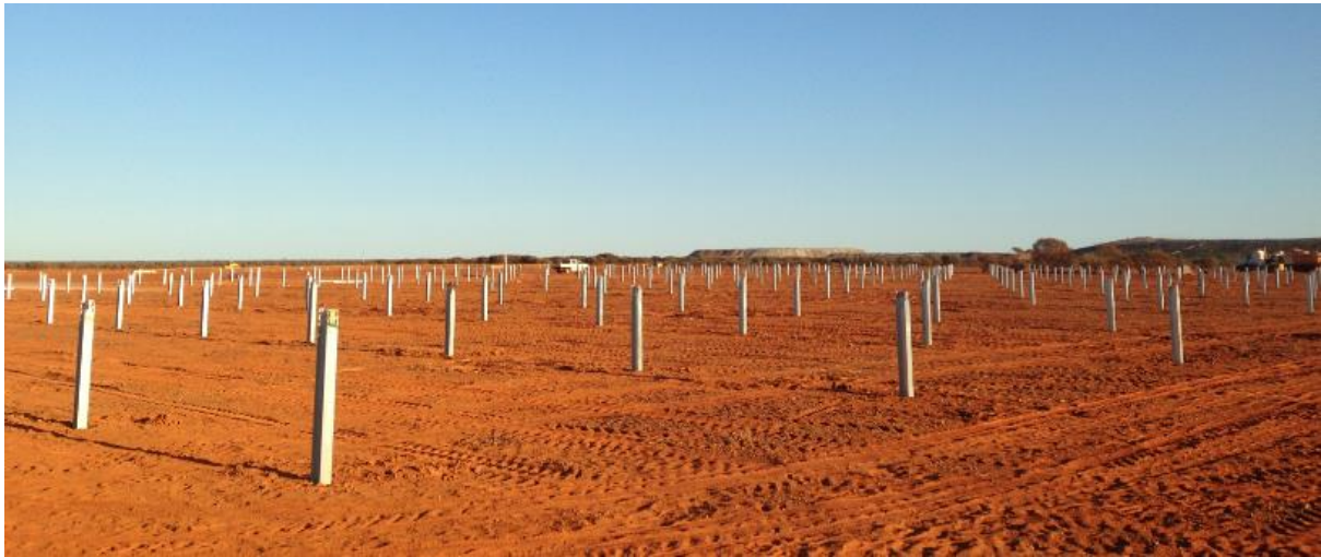
Figure 3-6 Example of poles driven into the ground on a Neoen solar project in Western Australia
