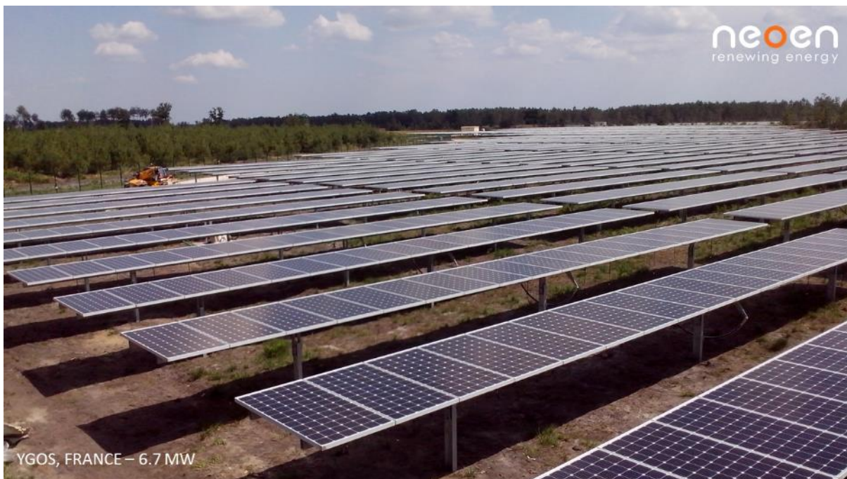
Figure 2-1 Example of single-axis tracking systems with multicrystalline modules
