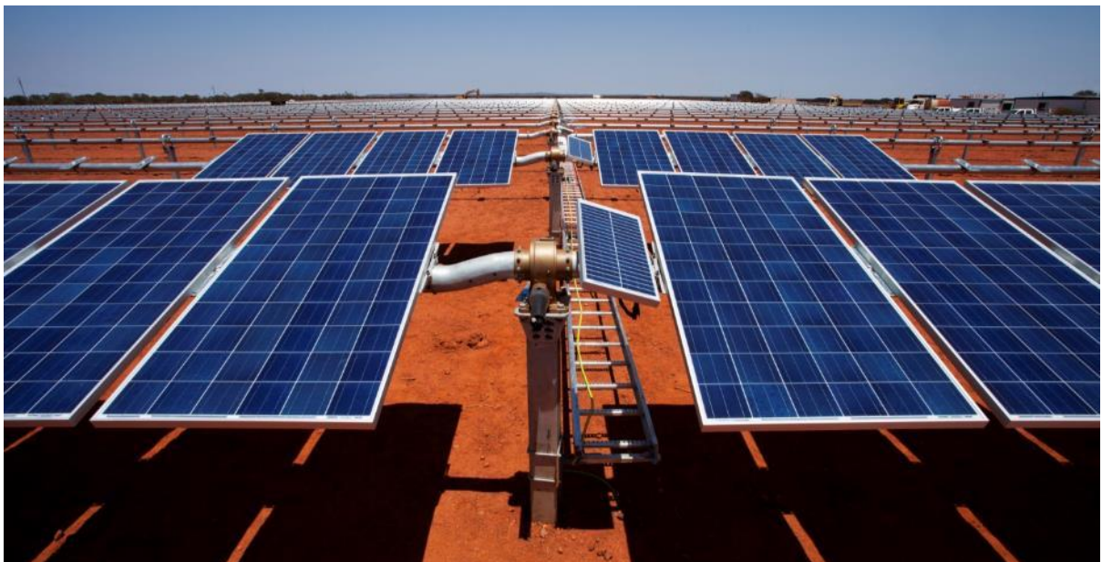
Figure 3-8 Example of a single-axis mounting system after panel installation
